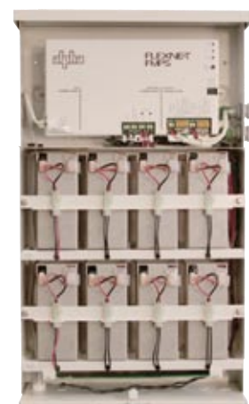
FMPS with cover removed and two 7.2Ah battery strings installed
